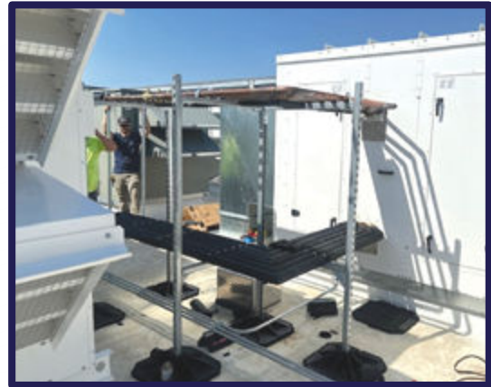
Air-to-Air Split loop energy transfer between 15 foot separated exhaust and supply air AHU's. Precool and preheat incoming air from exhaust AHU.
