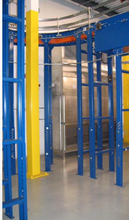
Figure 3: ATO-024 Located Under Mezzanine
