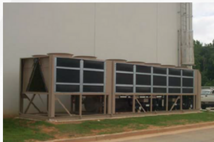
Figure 2: One of Two York 300 Ton Air Cooled Chillers
